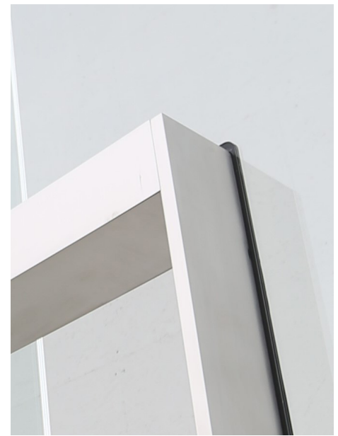
Figure 4. Notch in Glass Corner.
