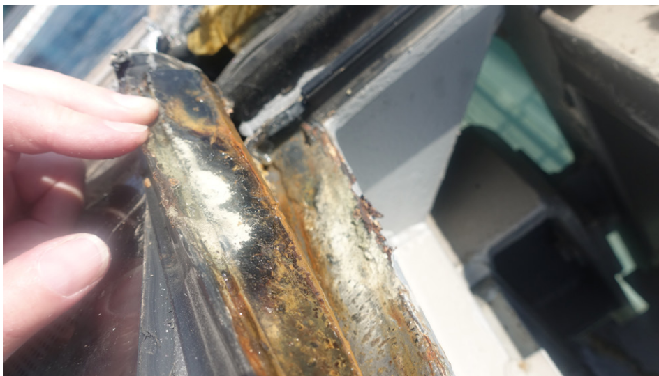
Figure 2: Unbonded crossing point with corresponding leaks and corrosion on the substructure.
